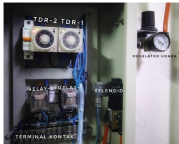
Gambar 4.1 Panel kontrol blow down
