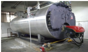
Gambar 4.1 mesin boiler merk “Tuff”
