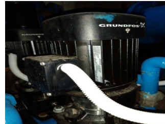
Gambar 4.7 Motor Pompa Air Grunfos
