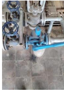
(b) Blow down manual
